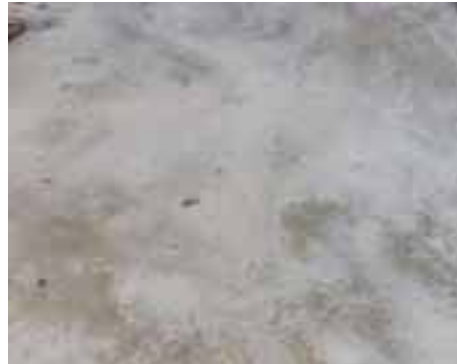
Before treatment, scale deposits formed on the floors and surrounding area.
